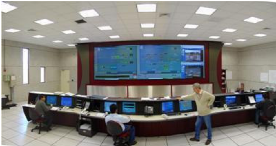
Figure 5: Camisea Pipeline Main Control Center
