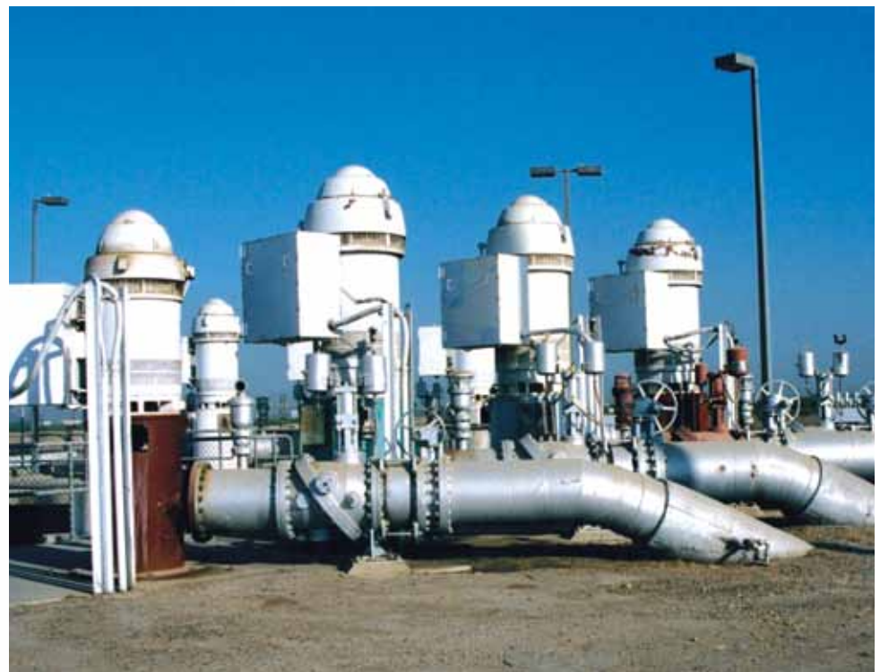
The system's three pump stations contain pumps ranging in size from 500hp to 1,000hp.
