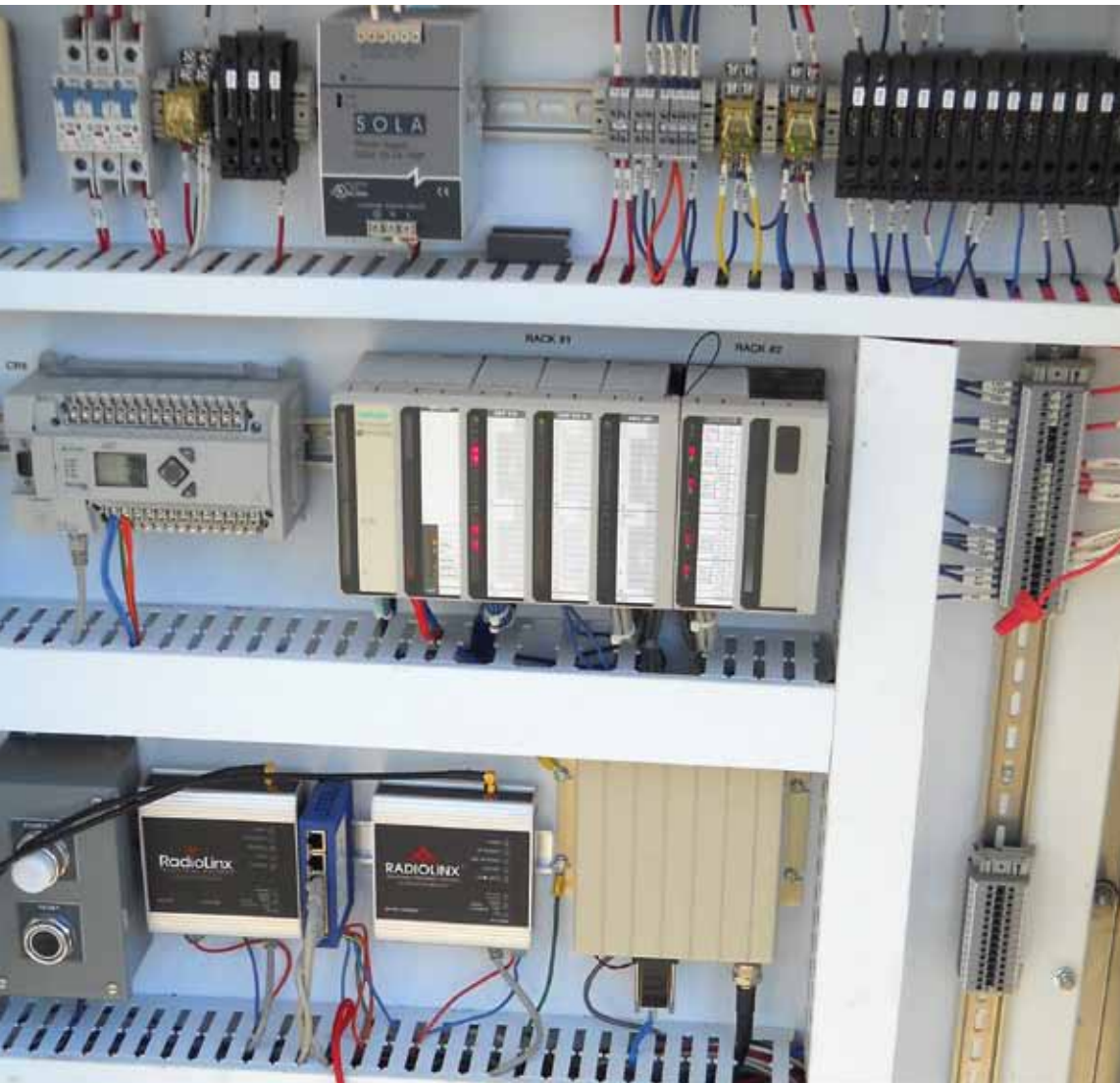
ProSoft Technology’s wireless radios deliver data fast for Padre Dam Municipal Water District
